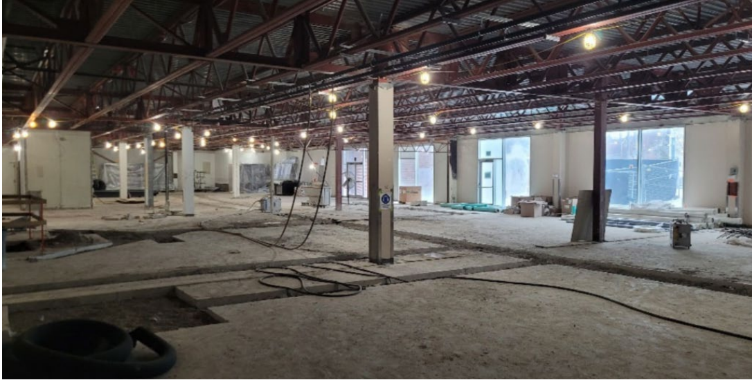
Ongoing work for installation of new services and structural connections – ZONE B
