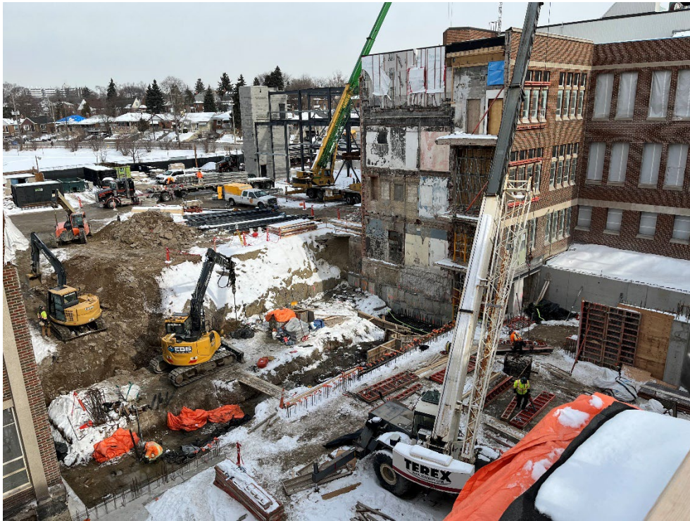
An overview of the auditorium helical pile installation, concrete foundations, backfill and grading – ZONE A
