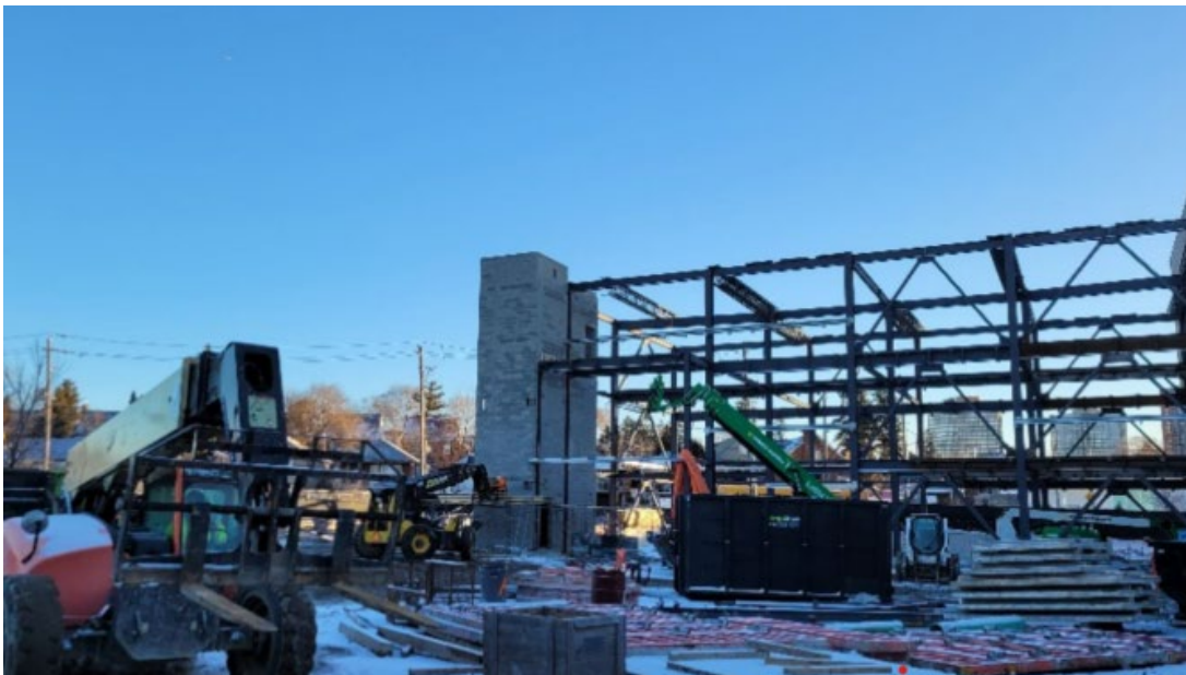
Ongoing structural steel erection and Stair J masonry block build up – ZONE C
