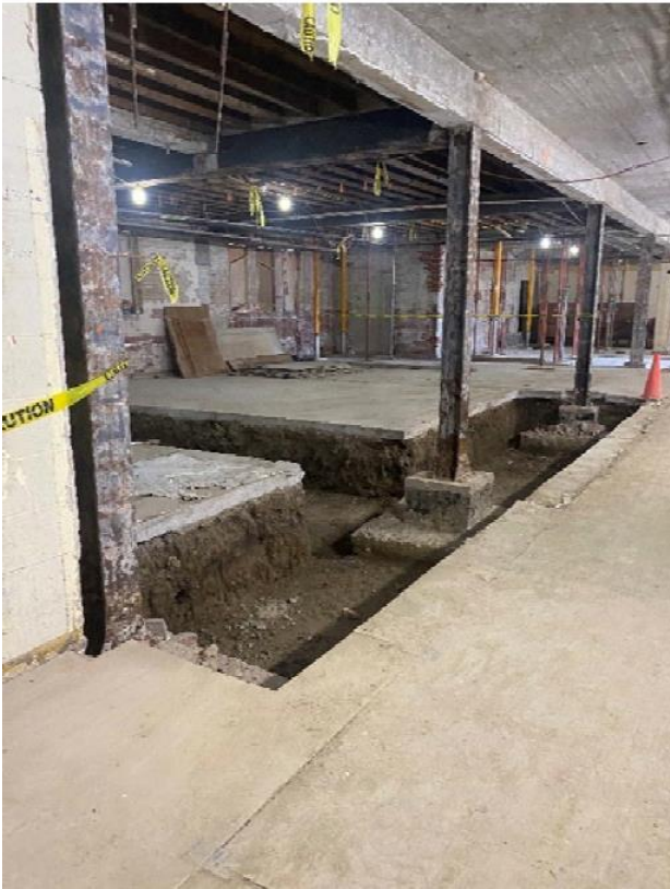
Exposed columns and soil conditions – ZONE A
