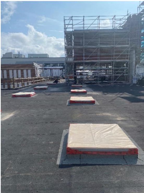
Pockets cut in temporary roof for new third floor steel column splice connections to existing second floor columns – ZONE A
