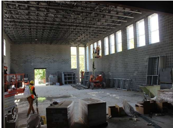
Interior photo looking to the west side of the new gymnasium from the stage showing window frame installation.
