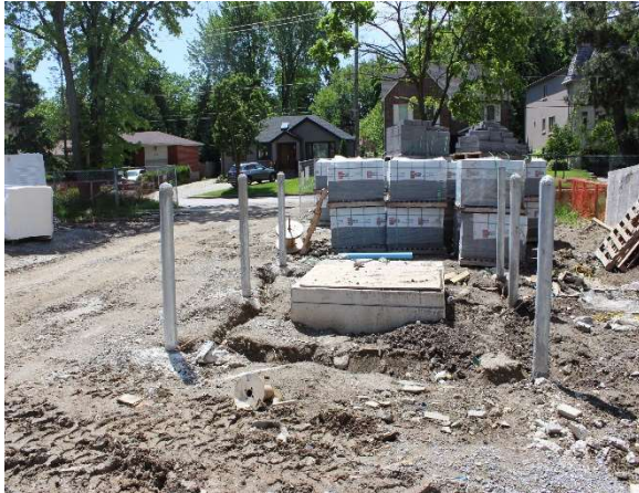
Exterior photo of completed hydro transformer pad ready for the new transformer.
