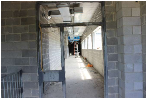
Photo of the east/west corridor of the childcare & classroom wing on the second floor from the stairs. This photo shows installed door frames and above ceiling mechanical & electrical rough-ins continuing.
