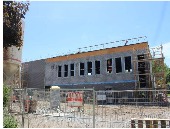
Exterior photo of the North elevation of the gymnasium wing showing window frame installation and progress of exterior façade.
