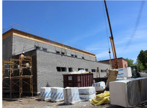
Exterior photo of the east elevation of the wing showing progress of the exterior façade.
