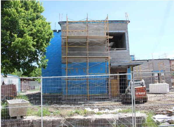
Exterior photo of the West elevation of the childcare & classroom wing showing installation of vapour barrier.
