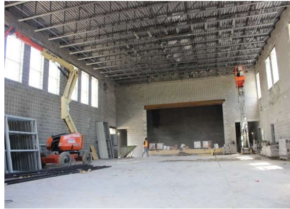
Interior photo looking to the east side of the new gymnasium showing the new stage.
