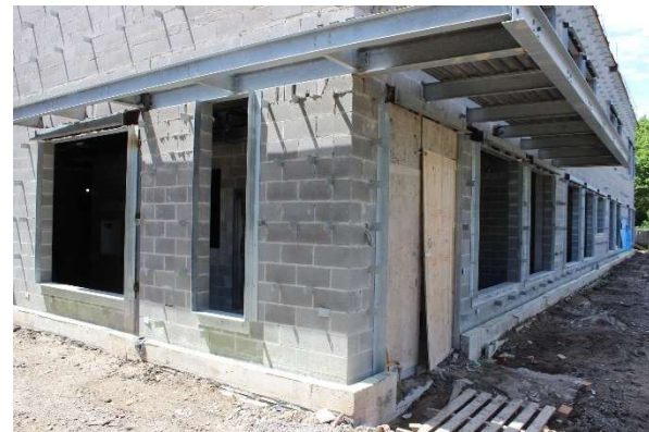
Exterior photo of the North-East corner of childcare/classroom wing showing the new childcare entrance with canopy framing completed and metal decking being installed.
