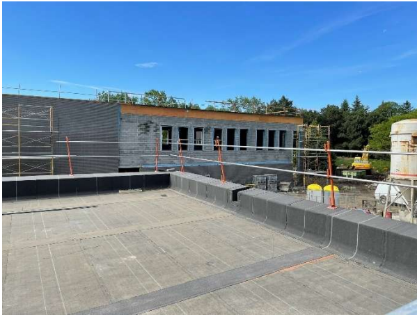
Exterior photo of roofing works on lower roof of the childcare & classroom wing looking at exterior façade of the gymnasium.
