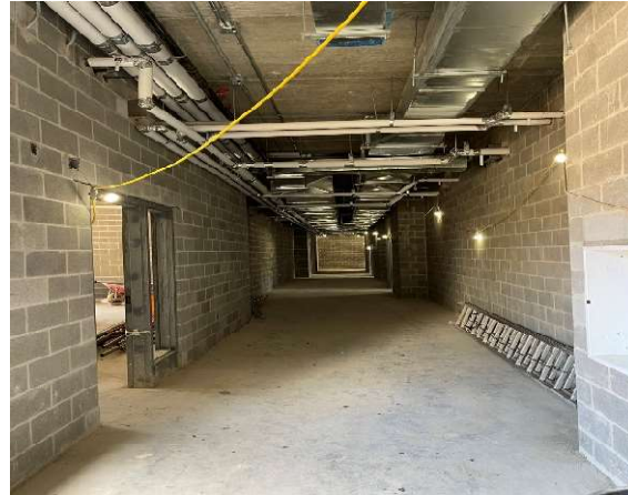
Interior photo looking down the east-west ground floor corridor of the childcare showing installed door frames and above ceiling mechanical & electrical rough-ins.
