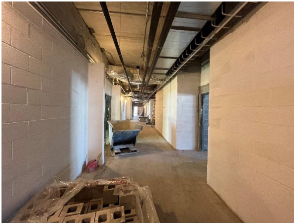
Picture looking down the ALPHA II Alternative school hallway. Rough-in are complete and block walls were recently primed.
