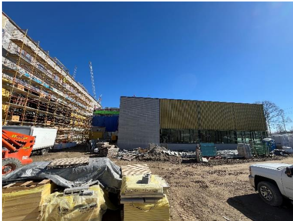
Picture taken from the South-West corner of the building looking at the Gymnasium. The exterior block veneer was recently installed.
