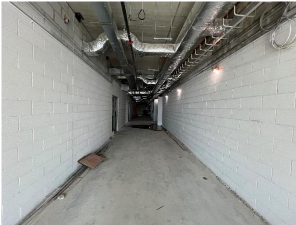
Picture of the hallway on the second floor. Rough-ins are about 95% complete and block walls were recently primed.
