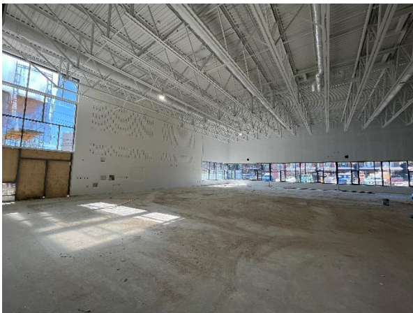
Picture of the gymnasium. Curtain wall glazing was completed a few months ago and the entire room was recently primed.
