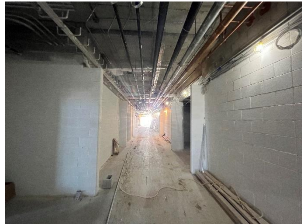
Picture looking down the North/South hallway of the first floor. Rough-ins have been completed for some time now and block walls were recently primed.
