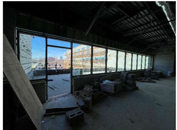
Picture from third floor hallway looking at the outdoor learning roof. The roof membrane was installed a few months ago.
