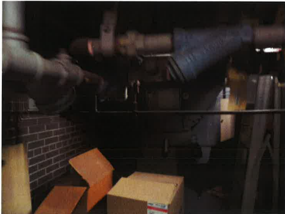
Photograph 4: View of the HVAC mechanical room
