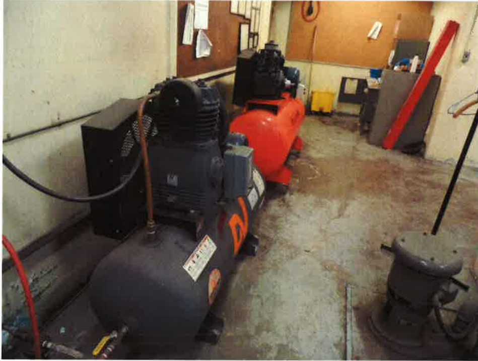
Photograph 7: Two compressors on the left and sump pump on the right. These units are located in the sub-basement.
