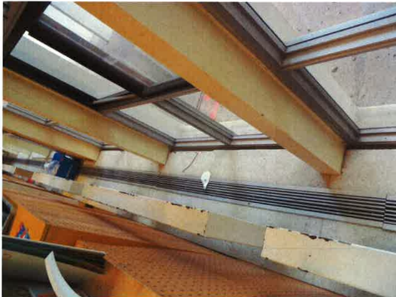
Photograph 10: Baseboard heating in one of the classrooms
