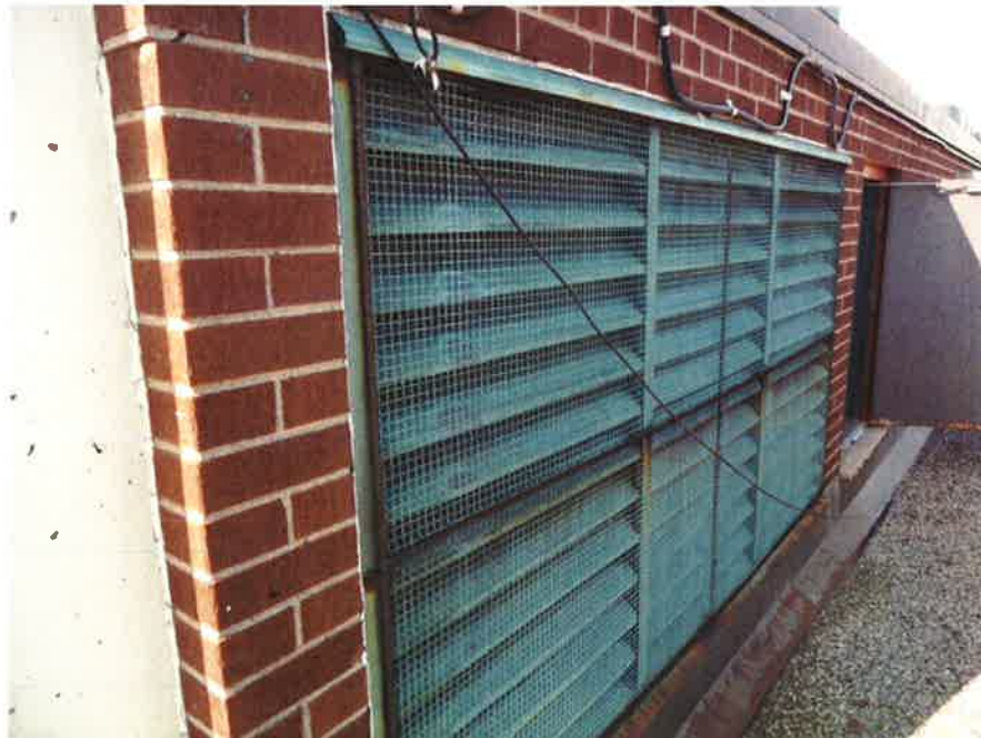
Photograph 2: Facing Southwest: Intake for conditioned air
