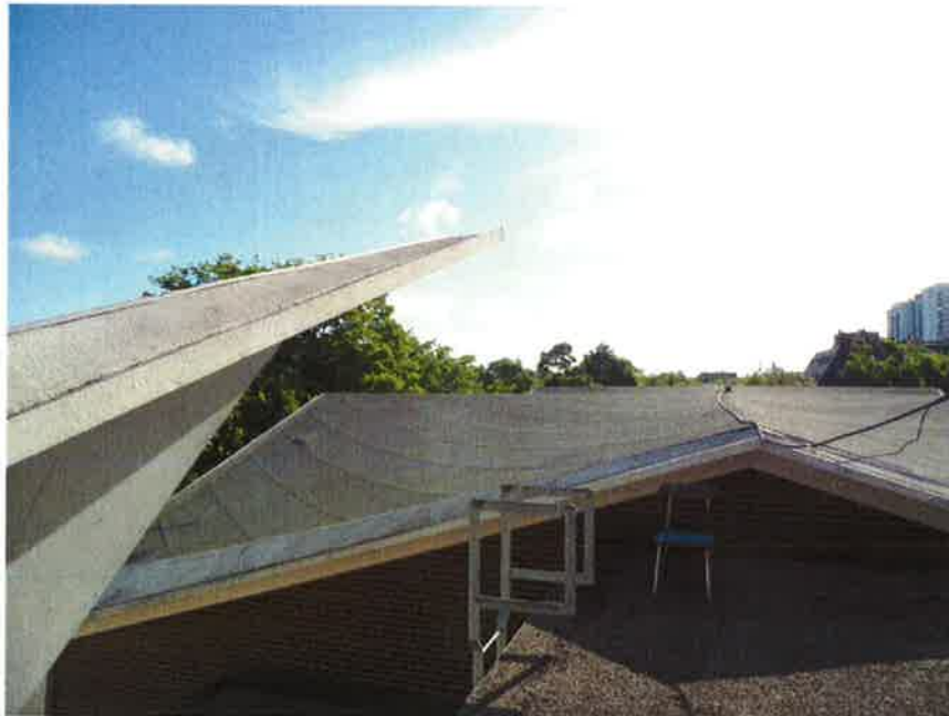
Photograph 12: Additional roof top photograph showing the uneven layout, therefore there are no rooftop units.
