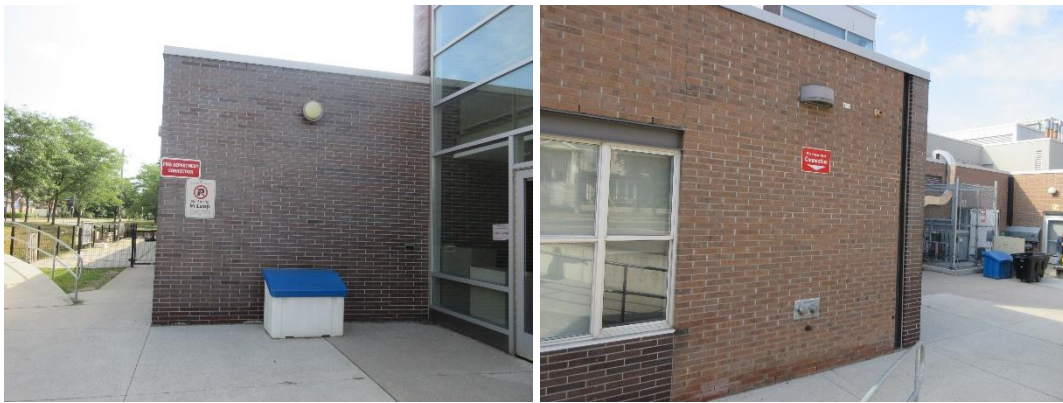
North Façade- Fire Department Connection
