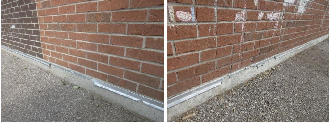
Damaged flashing at grade
