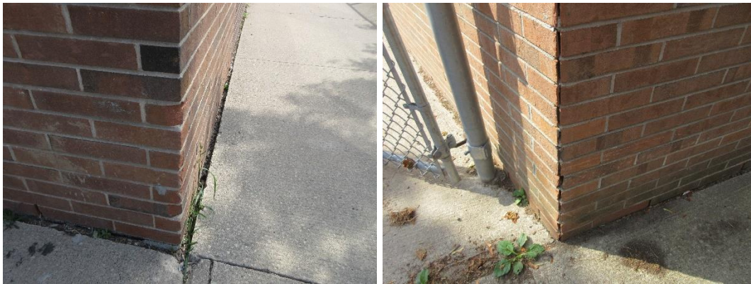
Brick conditions- chipping at corner joints
