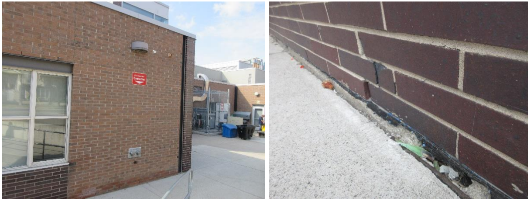
Brick conditions- deterioration/ damage at grade
