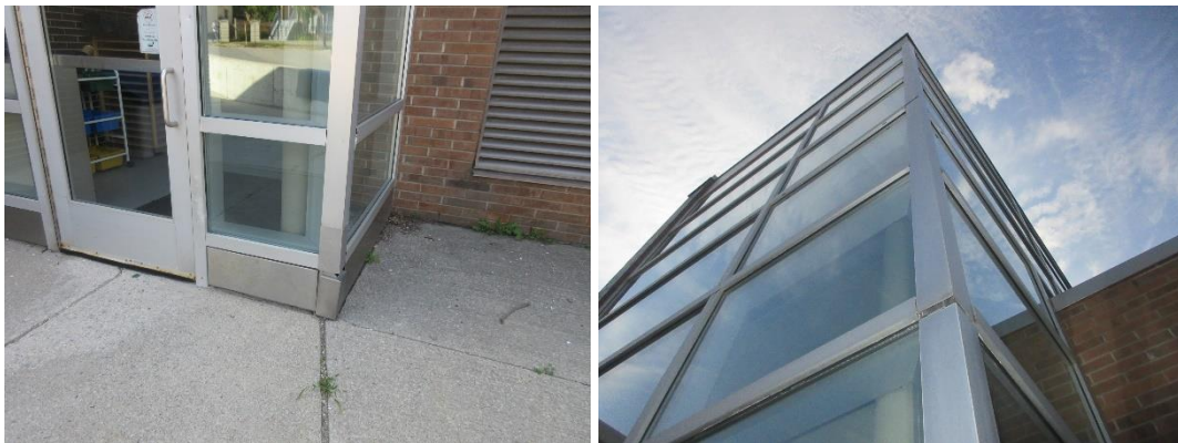
Alum. Curtain Walls & Doors- Minor damages & gaps between pressure caps
