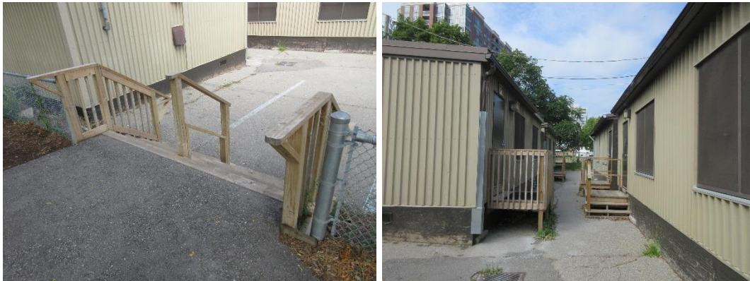
Portable Classrooms not accessible
